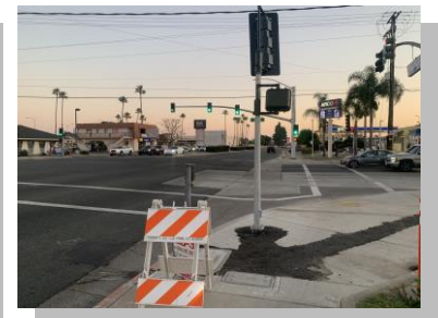
Brookhurst Street: New traffic signals were installed during the third weekend of January 2025.
