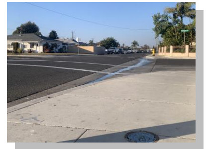
n°. 1 - Water in a cross pan where Riata Street intersects Madison Avenue (Midway City, California)
