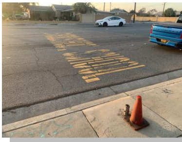
Goldenwest Street: “SCHOOL” markings on each lane, next to sign post base for a school speed limit sign that has been missing since 2022.
